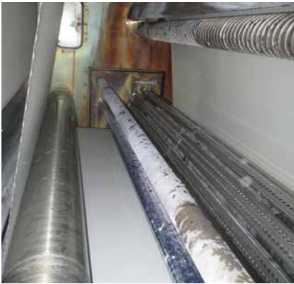
Segmented roller guider system SWS97 in bleaching steamer
